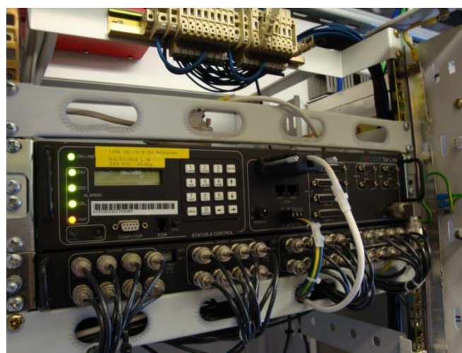
Figure 2: PCOM IDU, frequency independent IDU with 16 x 2Mbps ports (tribs) - split mount systems (IDU/ODU) (mid 1990s)
