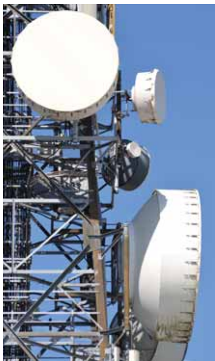
Figure 5: Microwave antennas in use at an operational mobile network operator's core switch site
