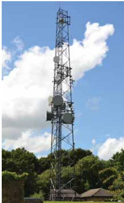
Figure 1: Point-to-point microwave radio hub site
